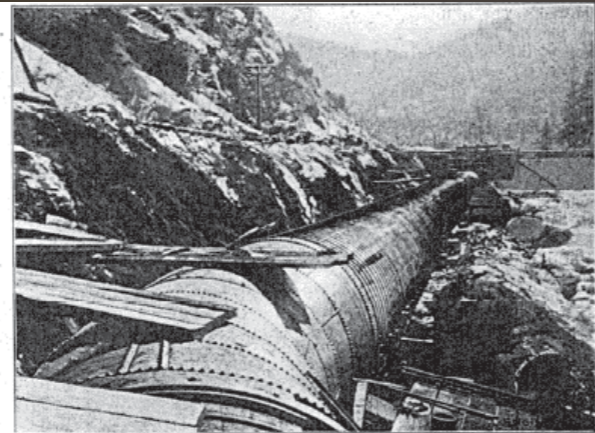
FIG. 2.—RIVETED STEEL ELBOW IN 9-FT. REDWOOD PIPE, NEAR FLORISTON, CAL.
